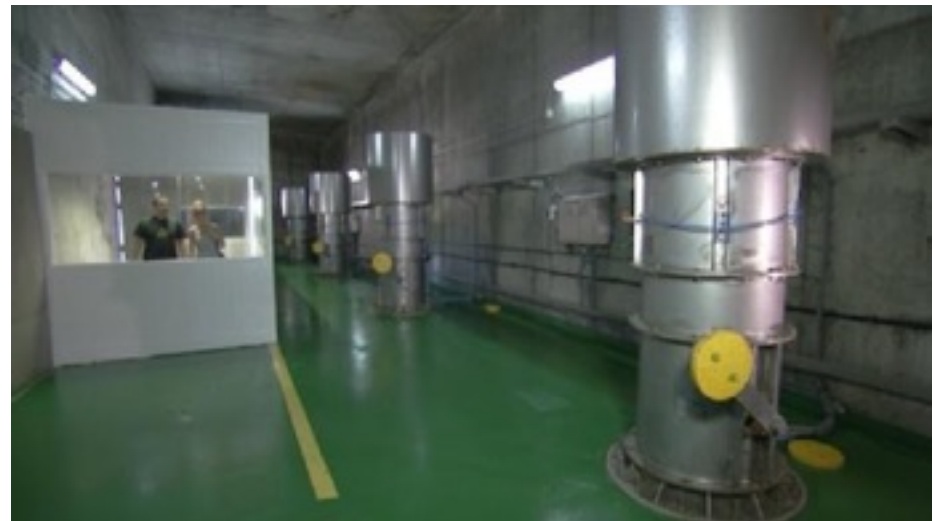
Mutriku turbine hall with public viewing booth
