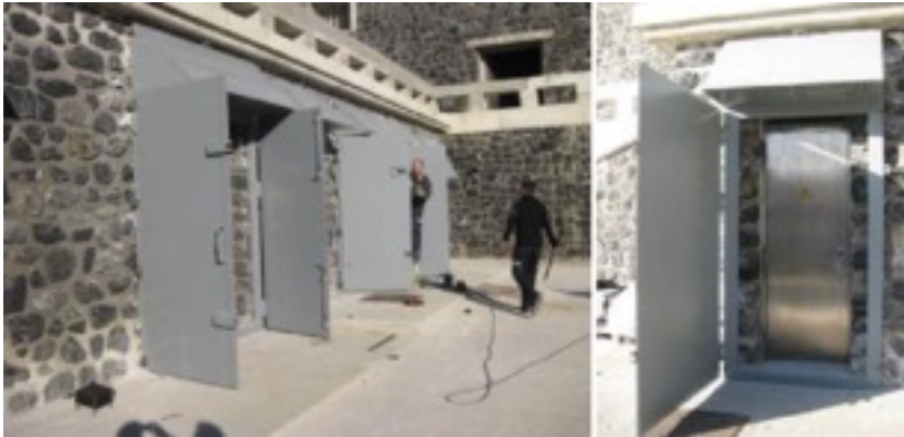
Mutriku control room protective outer doors
